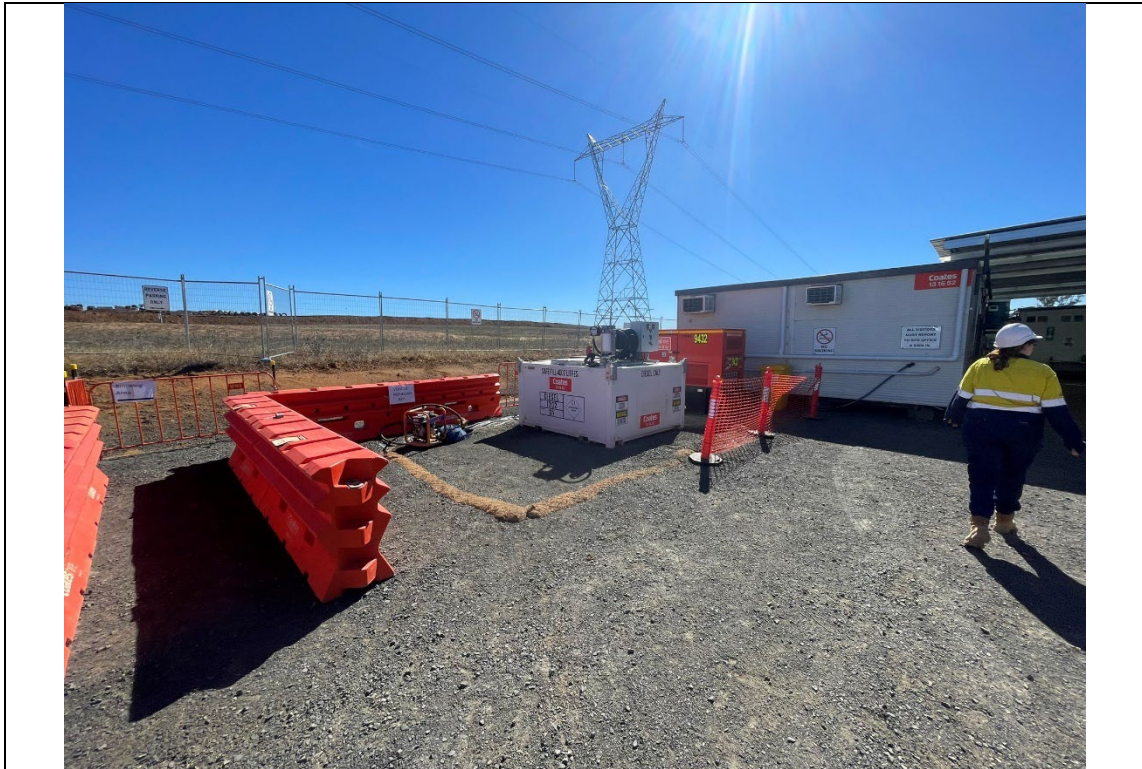
Photo 14 | Transgrid compound, diesel AST in bunded location.
