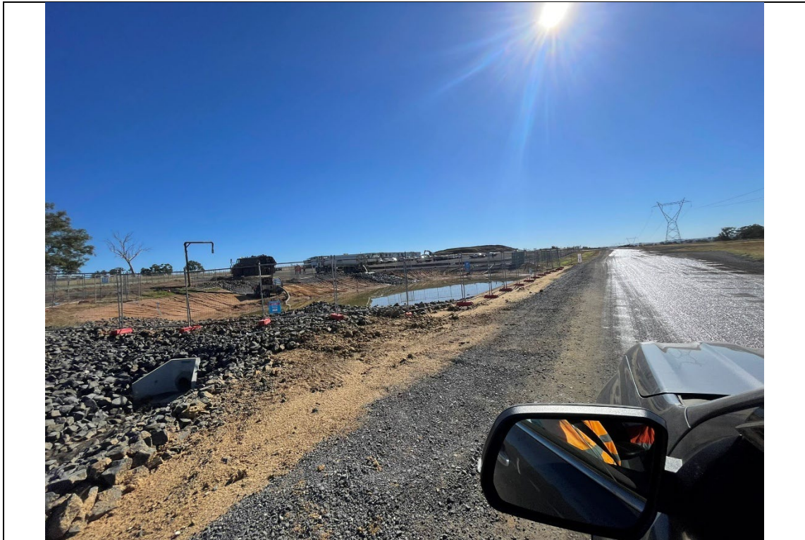
Photo 4 Onsite sediment basin installed as per ECP requirements and used to store non-potable water for onsite water cart refilling.
