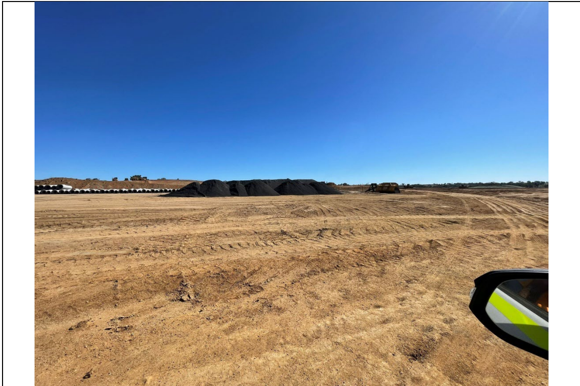
Photo 8 Samsung BESS cut and fill site. Surfaces being kept wet with no visible dust.
