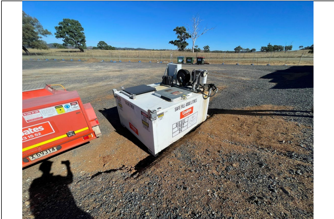
Photo 6 Above-ground diesel storage tank used to refill the generator.
