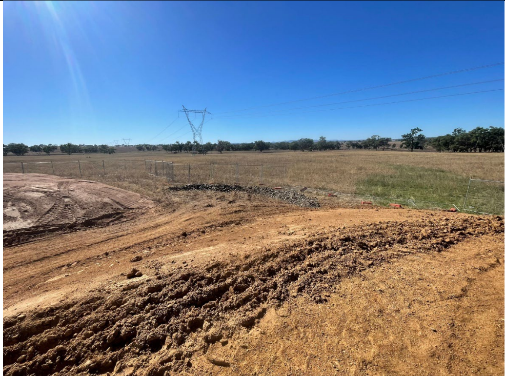
Photo 11 Samsung BESS cut and fill site, showing absence of sediment fence.
