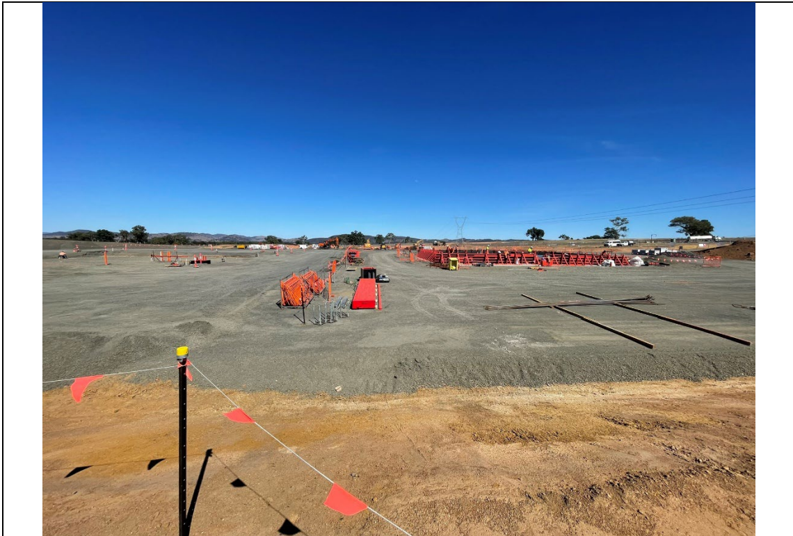
Photo 18 | Transgrid site, mostly sealed surfaces in preparation for substation installation works. Steel fixing works in progress.
