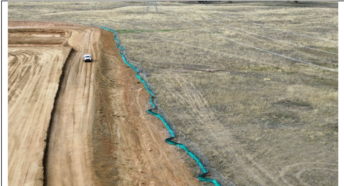
Photo 12 Samsung BESS cut and fill site, showing new sediment fence installed within 48hours of the audit inspection.
