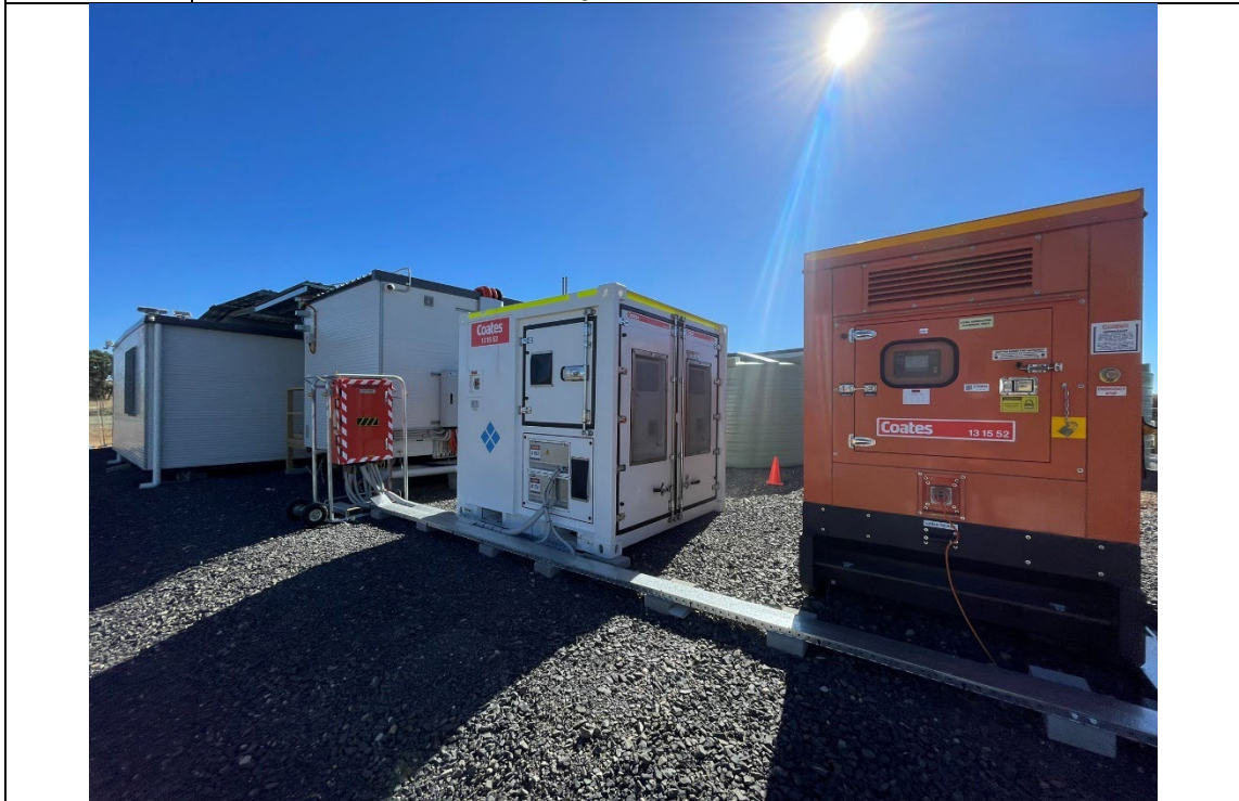
Photo 5 Generator and batteries to provide off grid power to the Samsung compound.
