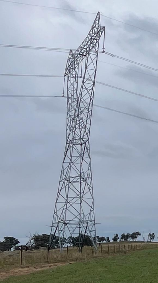
Photograph 6.1 Existing 330 kV transmission tower (tower 150) looking north
