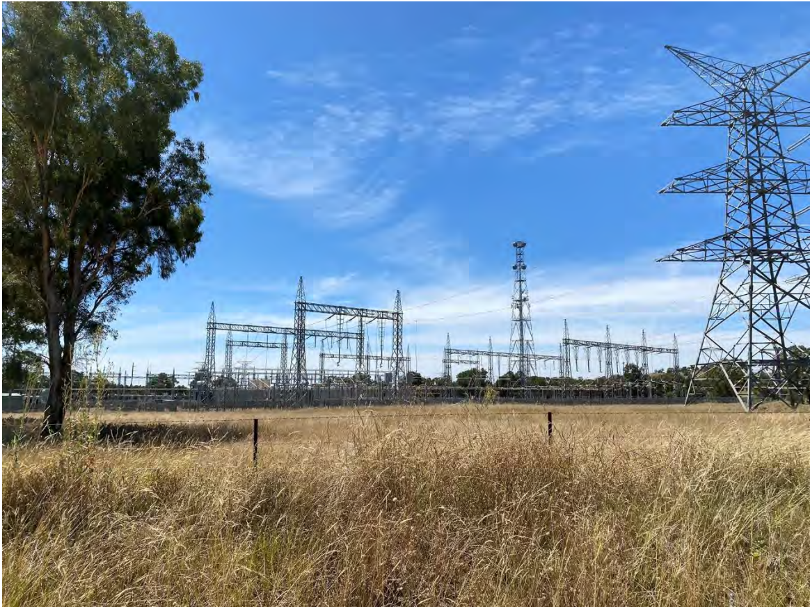
Plate 2-1: Transgrid Wagga Wagga 330kV substation
